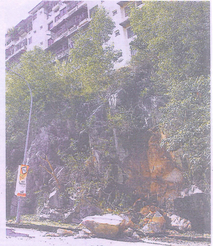
A common sight after a downpour: Taking care of the environment, even to ensure landslides do not occur, is everyone's responsibility. If the laid-back attitude is to continue, things will get worse like this rockslide that occurred after a downpour in Taman Bukit Permai in the Klang Valley recently.
